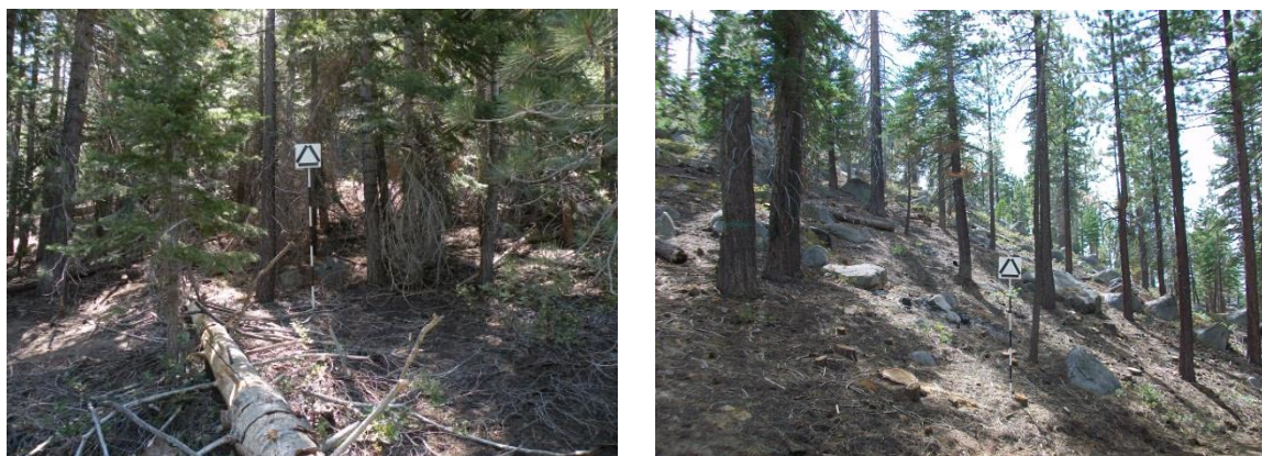
Figure 11. Hazardous fuels reduction to reduce the risk of extreme fire behavior (before and after)
